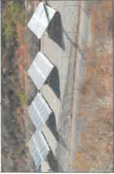
MJM Pump Station - 30kW
